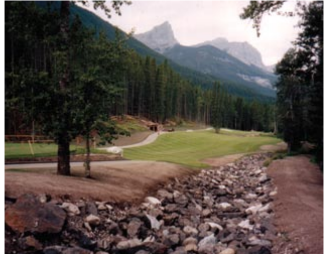
An early client success: Norwest's innovative designs to stabilize old underground workings also resulted in the development of a new golf course.
